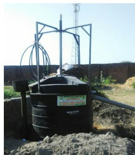
Installed HDPE Gobar Gas Plant at Farmers Field
