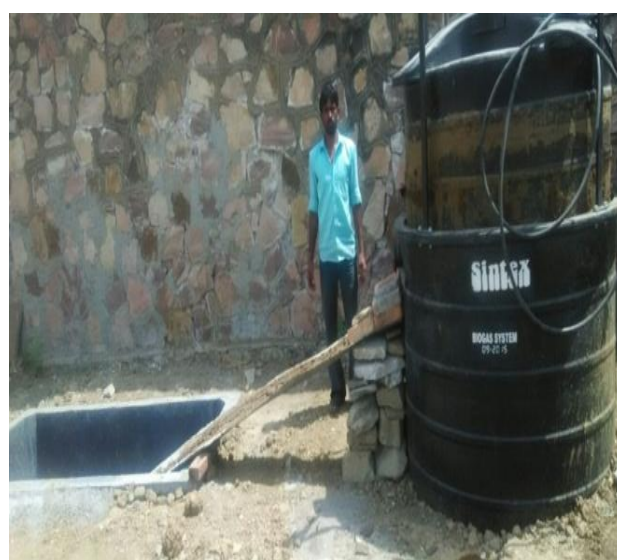
Biogas Plant with Slurry Tank
